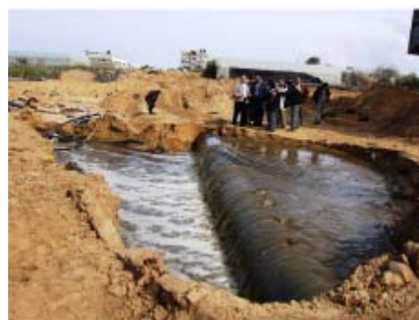
Waste water facilities damages, picture provided by CMWU
