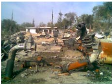
Water well damages, picture provided by CMWU
